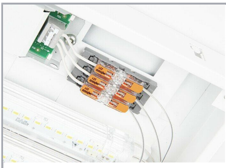
Multi-pole, fixed lighting fixture wiring
